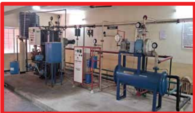
Thermal Engineering Laboratory
